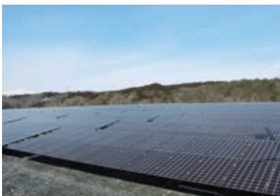
Kurihara Solar Power Generation Plant of the Company (Miyagi Prefecture)
